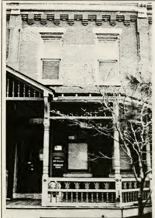
Figure 8. 628 Benson Street Camden, NJ. Inappropriate repointing on the front elevation of the building.
